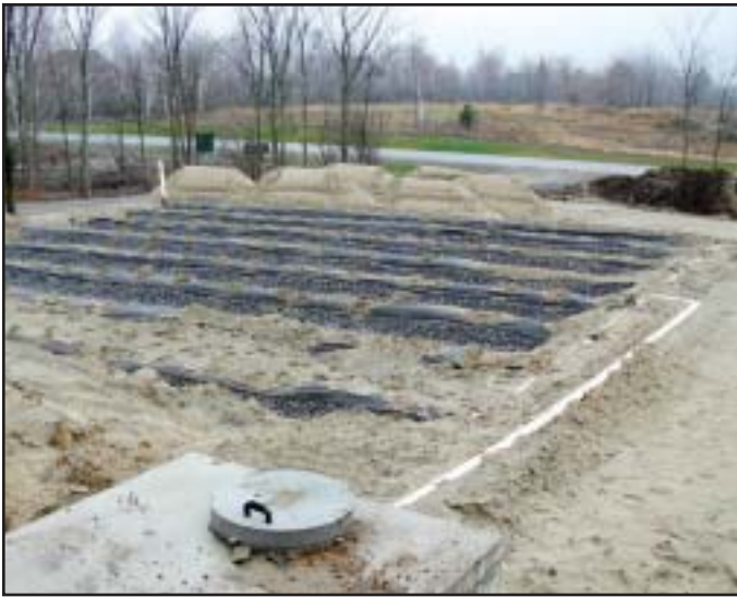
Leaching bed with perforated PVC drain pipes.
