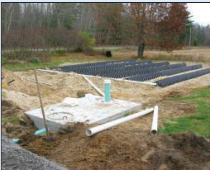
Leaching bed with gravelless trench technology.
