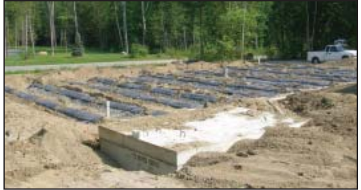
Septic tank and leaching bed.
