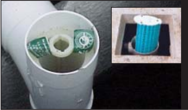
Effluent filter in septic tank.
